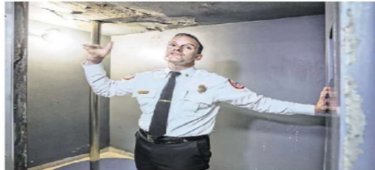
Miami Fire Chief Robert Hevia tours Fire Station 1, where mold, water intrusion and outdated equipment are hampering responses and community safety, during a press tour.
