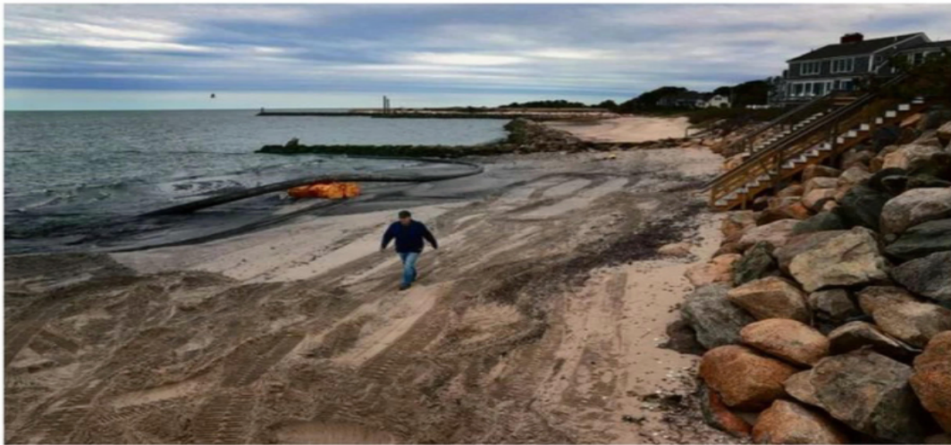
Ken Cirillo, dredge director in Barnstable County, walked along a beach in Harwich where new sand was being added.
